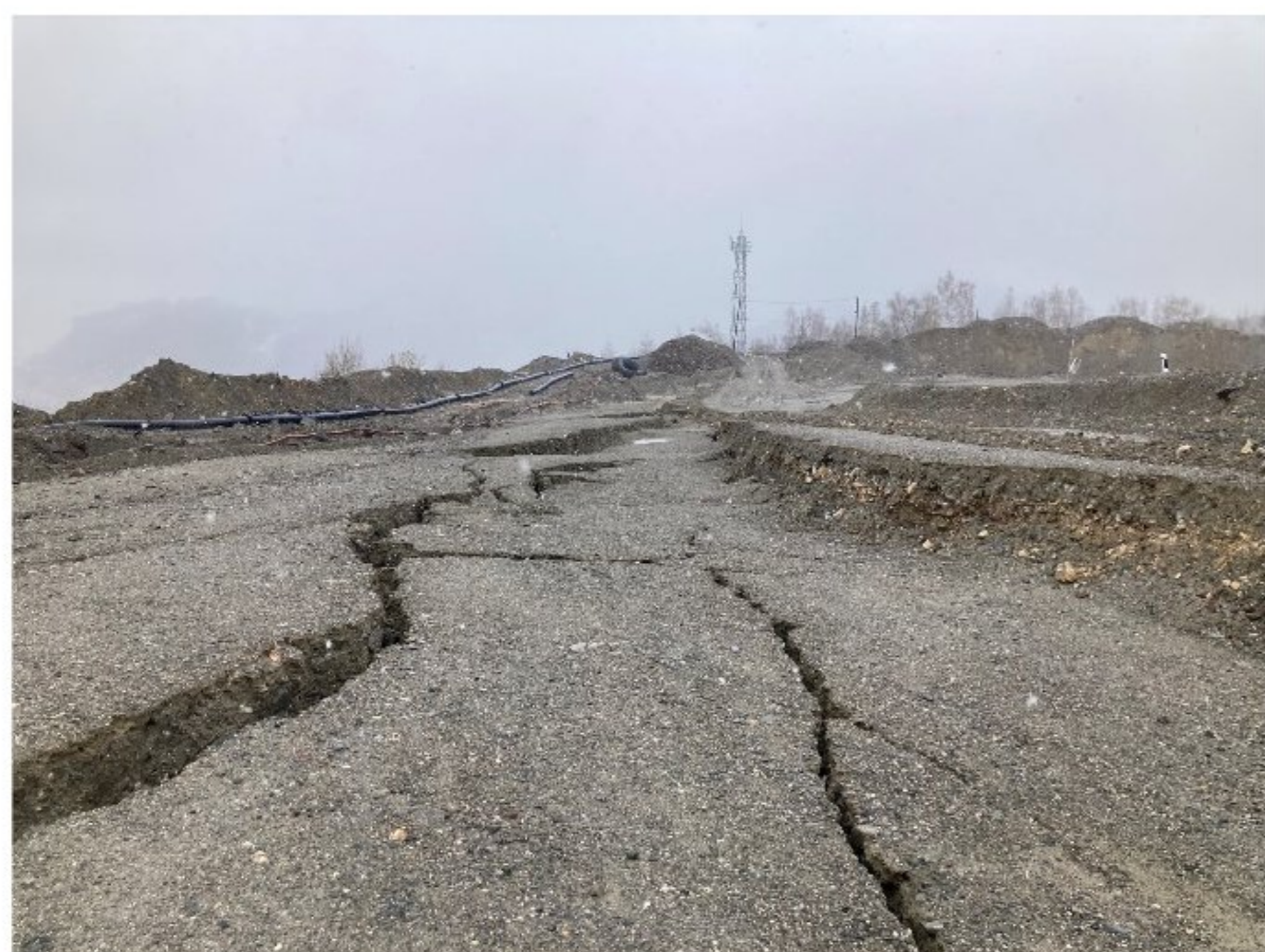
Figure 2 Gapping cracks and local benching between conjugated failure planes on the abandoned tailing horizon 550 m.
